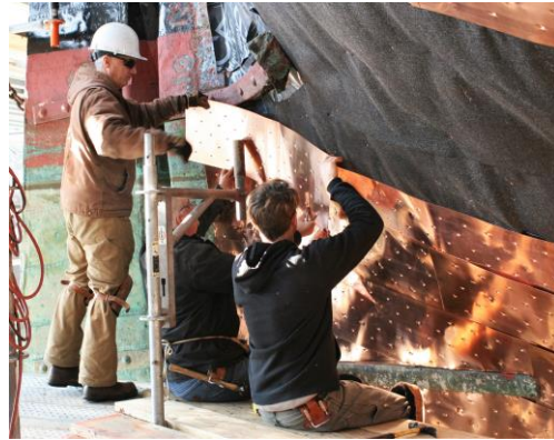
Copper sheathing installation by David Cavanaugh (left,) Joseph Halter (center) and Bruce Caporal (right) just forward of Constitution's rudder, starboard side, February 2017 15
