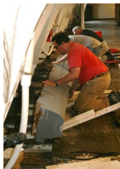
Ian Robertson (foreground), Alex Briere (middle) & John Pelikan installs port gun deck waterway, August 2015
