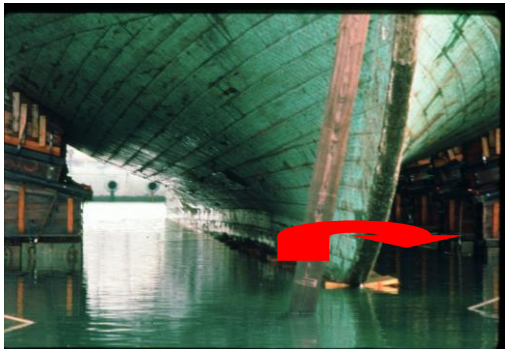
Constitution ’s 1795 keel with a 14” hog at the beginning of the 1992-1996 restoration, in Dry Dock 1
